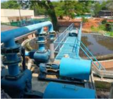
500 KLD STP at Kozhikode medical College
