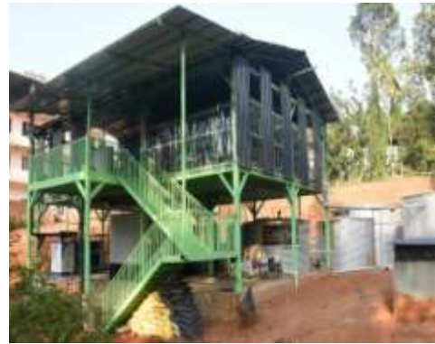
1 MLD STP at Kozhikode medical College
